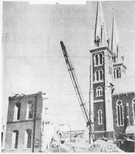
UNIQUE VIEW—This is the first published photograph of the full expanse of the majestic spires of St. John's Church, Indianapolis, as viewed from the south. The demolition of the old St. John's grade school, a segment of which is still standing at the left, made it possible for Criterion News Editor Paul G. Fox to get the historic picture. The demolition work has now been completed, and construction is starting on a new three-story Archdiocesan office building.
