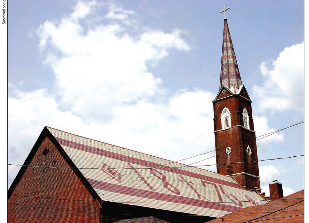
The new slate roof installed on St. Mary of the Immaculate Conception Parish in Aurora last summer bears an exact resemblance to the prior slate roof that lasted more than 100 years. For its role in preserving the roof, two historical foundations have given the parish awards.
