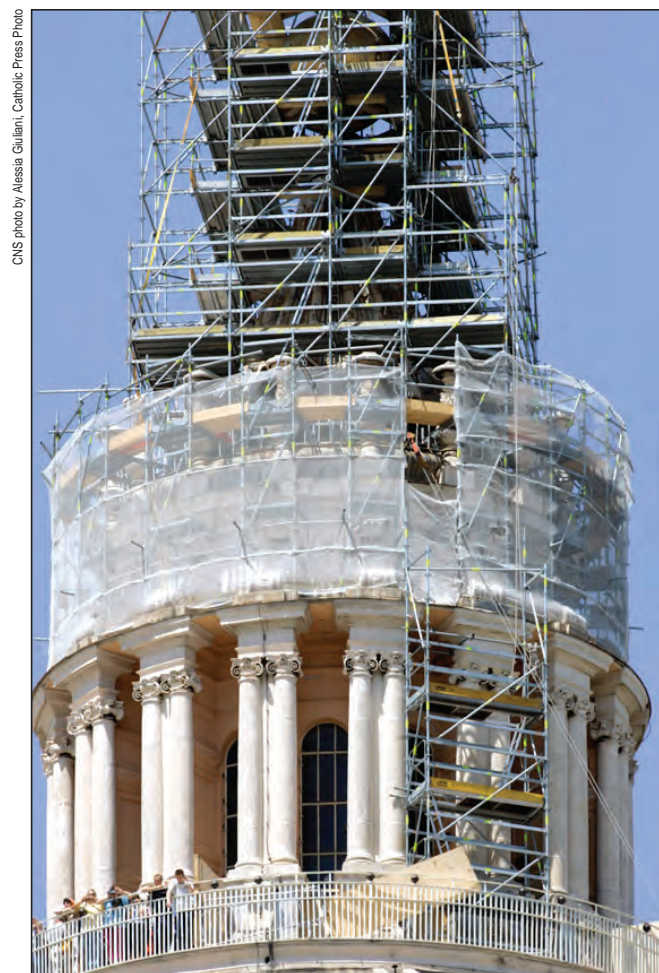
Scaffolding is seen on the highest part of the dome of St. Peter's Basilica at the Vatican on June 16 as workers restore the lantern and the gold-coated bronze sphere on top of the dome.
