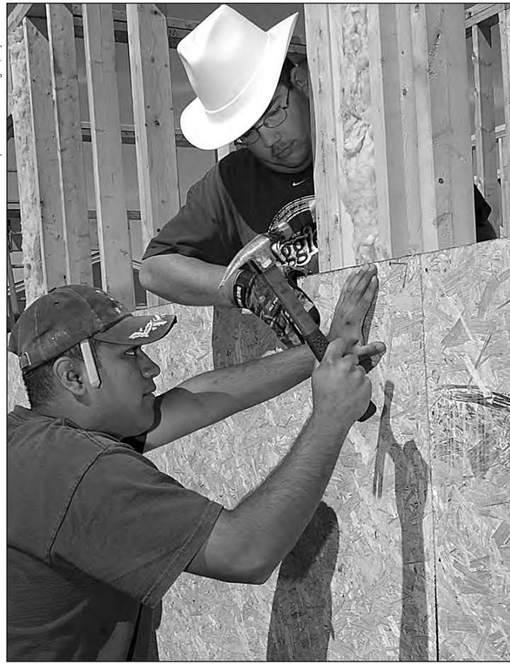
Richard Sanchez hammers a nail on March 17 into sheathing while John Hage holds the sheathing in place on one of 50 homes that Habitat for Humanity is building in Bayou Blue, La. The Bayou-area Habitat for Humanity is building the homes for families displaced by hurricanes Katrina and Rita. Both men are members of the Knights of Columbus from College Station, Texas.
