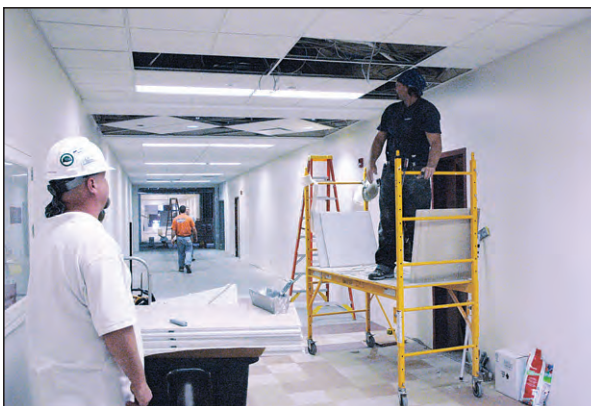
Construction workers make improvements in a hallway at Father Thomas Seccina Memorial High School in Indianapolis on July 23. The Indianapolis East Deanery interparochial high school is using a $1 million allocation of a Lilly Endowment grant to the Archdiocese of Indianapolis to make capital improvements.
