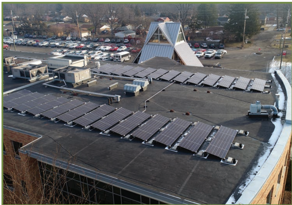
Solar panels sit on the roof of Cardinal Ritter Jr./Sr. High School in Indianapolis. In addition to reducing the school's carbon footprint and utility costs, the panels are being integrated into its science and theology lesson plans. (Submitted photo)
